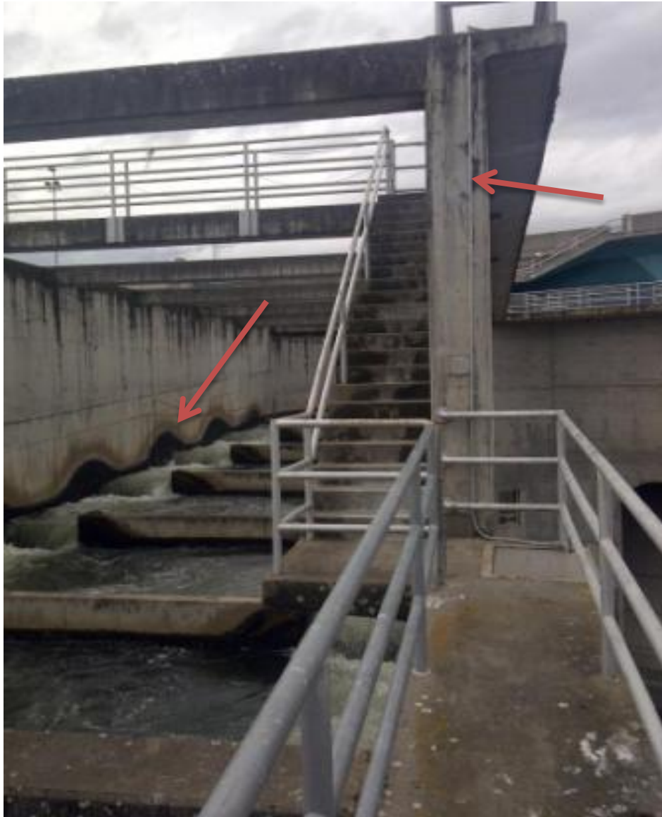
U of I electrical conduit installed upper east ladder for OSHA compliance Leading to half duplex antenna in background.
